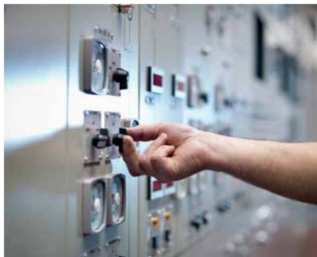
Central control room operation
