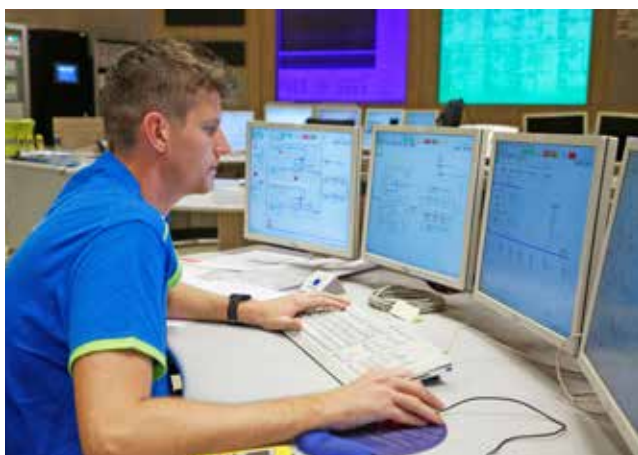
Central control room on the Flamanville 3 nuclear power plant
