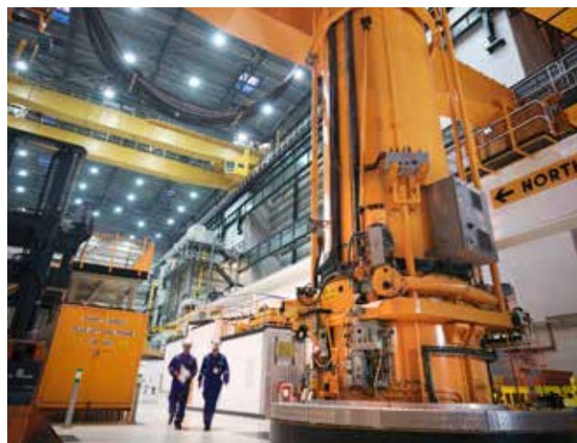
Refuelling machine at Hartlepool nuclear power plant
