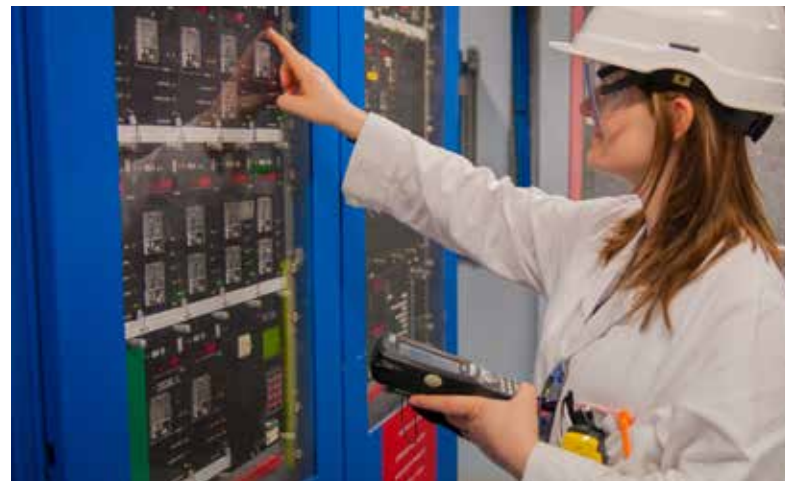
Reading parameters in the electrical switch rooms, Blayais
