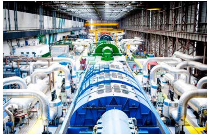
Turbine Hall, Tricastin
