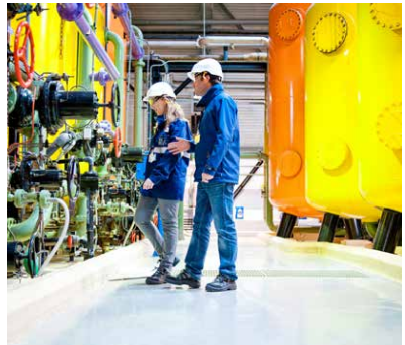
Technicians in front of the osmosis plant at Tricastin
