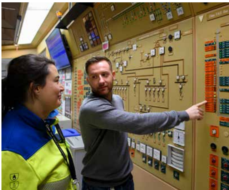
Main control room, Flamanville 1&2
