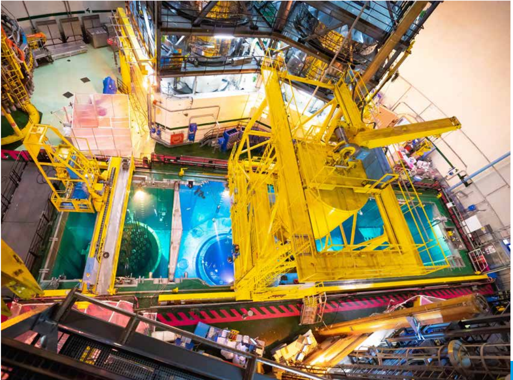
Cattenom – Reliability for a safe fuel handling operation
