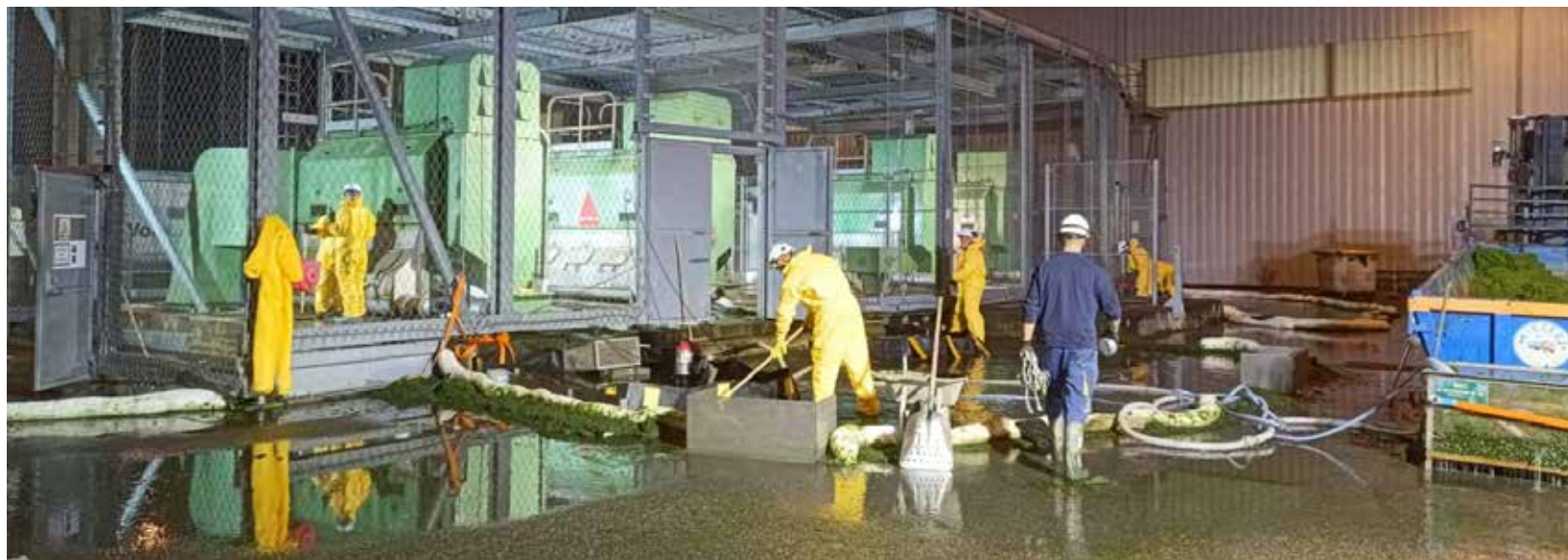
Chinon – Cleaning chain filters
