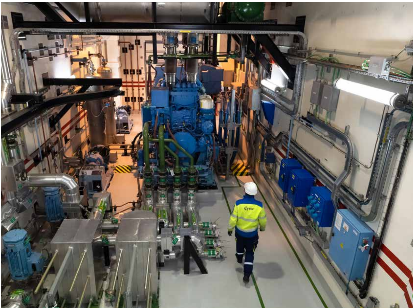
Flamanville 3 – Onsite electric power source diesel walkdown
