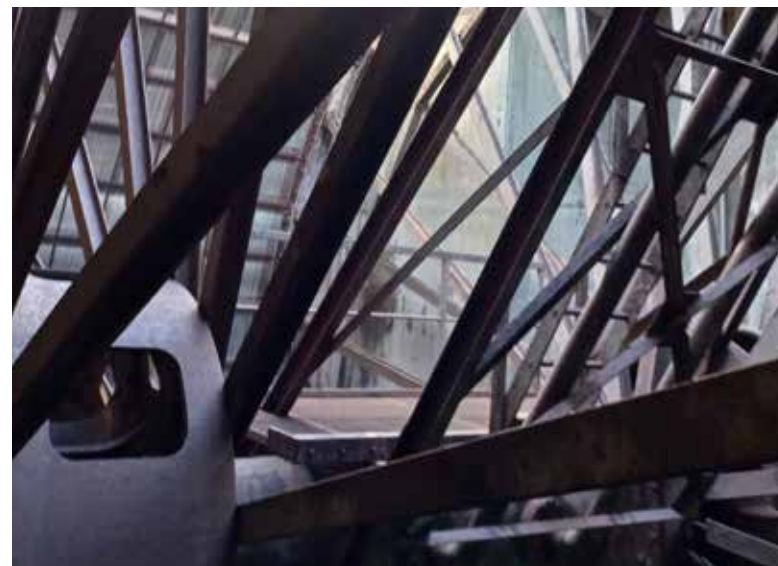
Bugey - Pumping station drum filter
