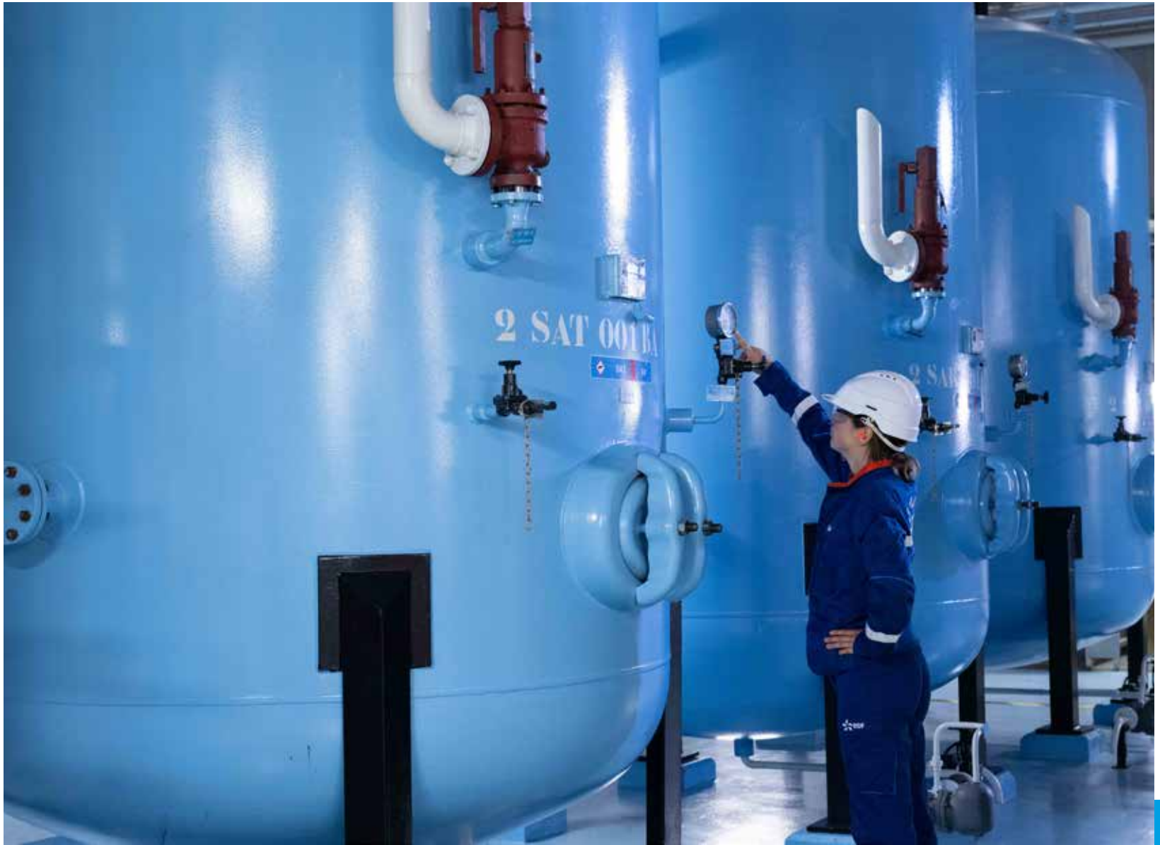
Golfech – Field monitoring of power generation equipment
