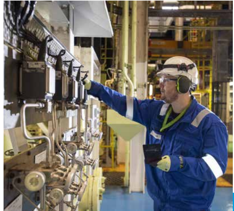
Hinkley Point B – Round in the turbine hall
